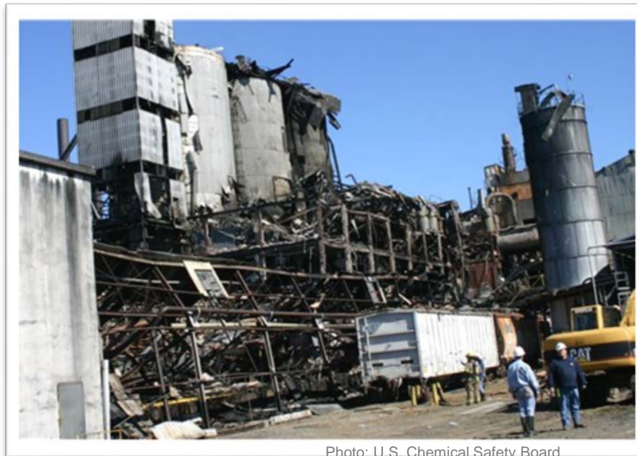
Photo: U.S. Chemical Safety Board
