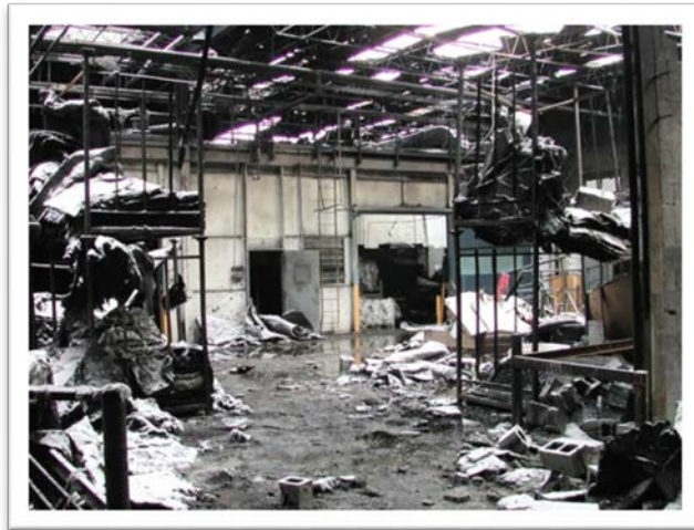
Photo: U.S. Chemical Safety Board
